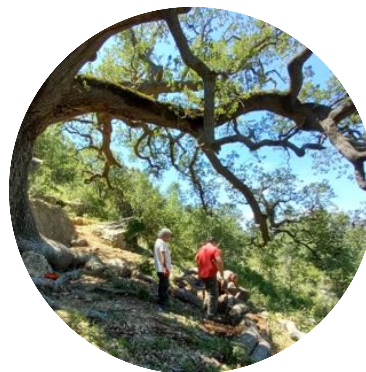
Construction of a wall made of branches interlocked with stones to retain soil and runoff water and prevent the passage of people, in «Roure de la Roca», in Barranc dels Horts (Ares del Maestre, Castellón).
